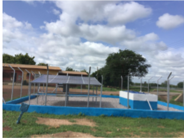
Photo 6: Solar Panels and Mechanized Pump at the Nangode Health Center.
