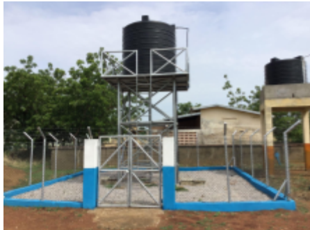
Photo 5: 10,000L Storage Tank at the Nangode Health Center.
